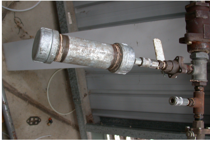
Figure 61: The ‘container’ connected to the brake pipe.
